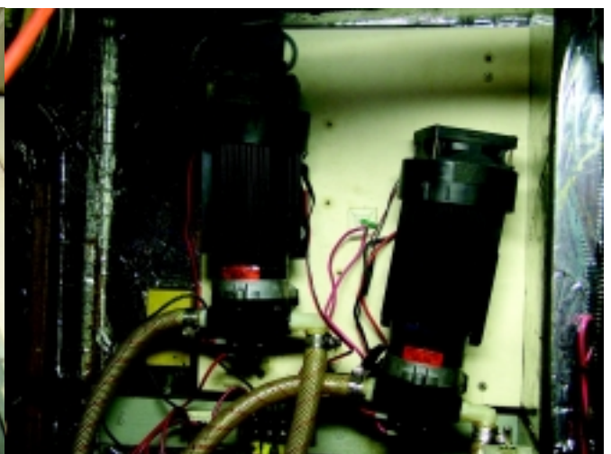
The system utilizes two 12-volt Shurflo feed pumps
