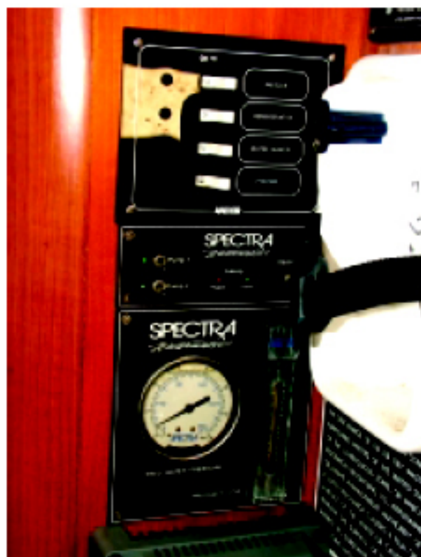
The control panels of the watermaker, above, and the Westerbeke generator, right
