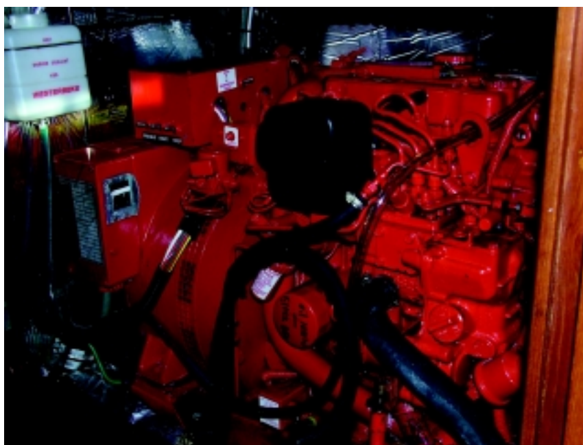
The author, opposite, charges his batteries with a Westerbeke generator, above
